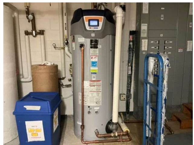
18 - DOMESTIC WATER HEATER
