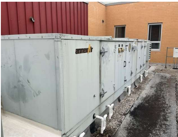
15 - ROOFTOP AIR HANDLER
